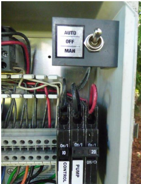
Figure 2 Typical pump controls (top) and circuit breakers (bottom) found inside control box.
