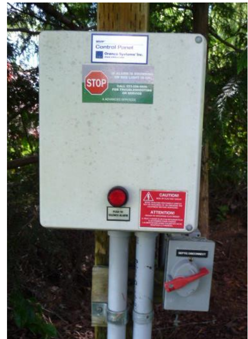
Figure 1 Typical septic tank control box with red indicator button (center) and main power switch (bottom right).
